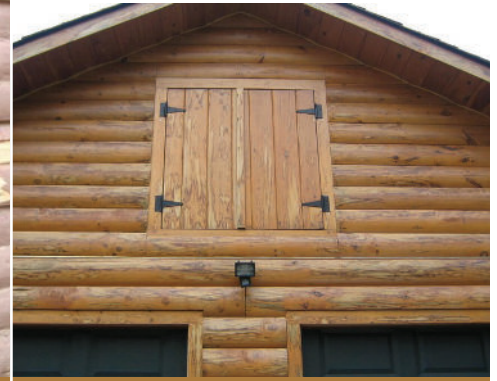
While water problems are never fun, a semi-transparent stain allows you to see developing problems, as shown with the tanning staining in this photo.
