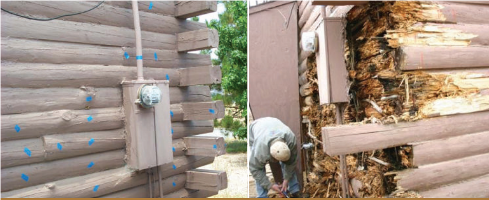
Note the blue tape on these logs. Those all mark areas of rotten wood. Before they knew it, they were digging out the entire corner of that house
