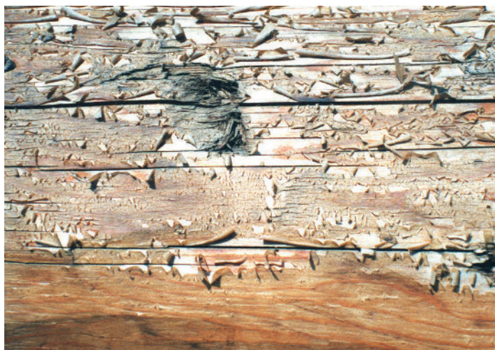
Too much water vapor pressure can result in stain that peels, as pictured.
