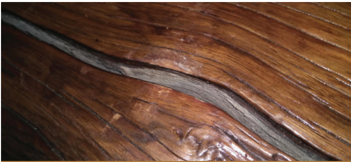
Checks and cracks like this can hold a lot of water and should be sealed to help prevent moisture infiltration.
